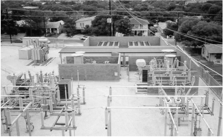
Fig. 1.29. HVDC Back-to-Back with Voltage Source Converters, 2 x 36 MVA (Source: ABB)
