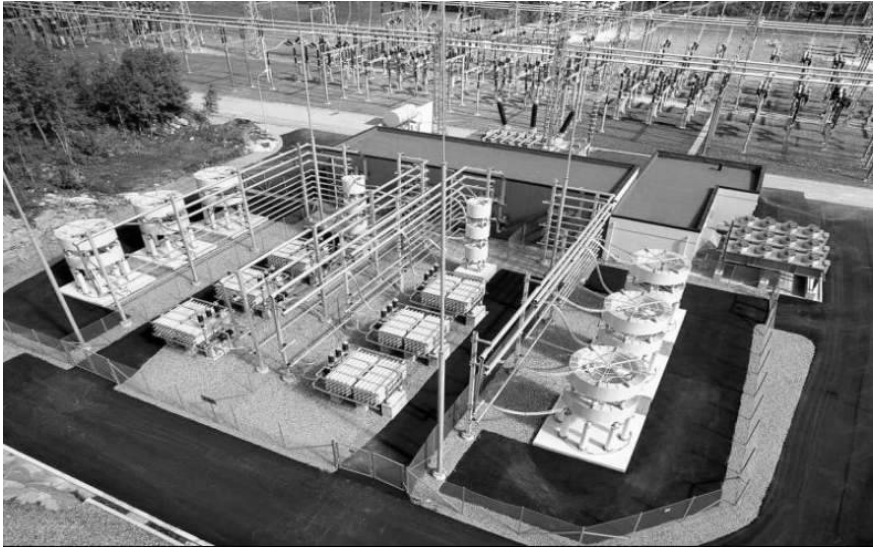
Fig. 1.12. SVC (Source: ABB)
