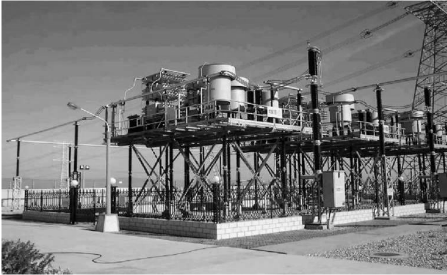
Fig. 1.17. Series Compensation (Series Capacitor) (Source: ABB)
